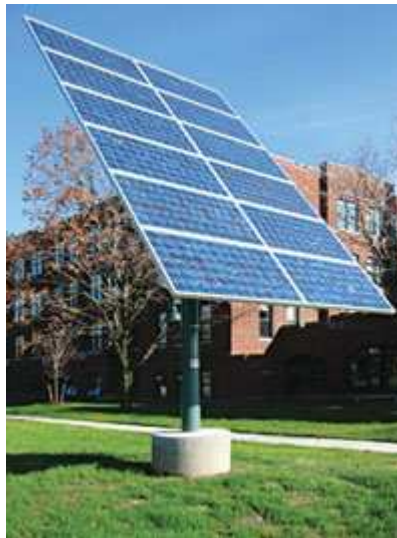
A photovoltaic array at Felician Sisters Convent, Coraopolis, Pa. The Franciscan nuns converted their 70-year-old provincial house into 10 household clusters of individual rooms with private baths. The renovation earned LEED-NC Gold certification. PHOTO: © ALEXANDER DENMARSH
